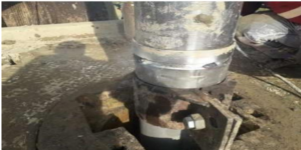
Figure 15: photo de tubage (Mohammed Ali)
